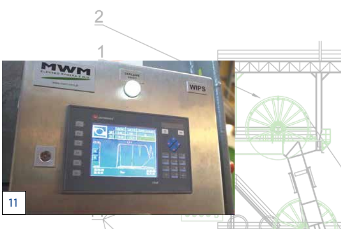
photo 11 – Vibrations monitoring system screen
